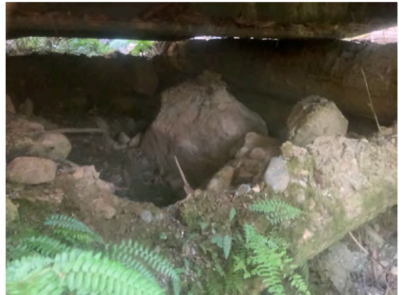
Right bank. Fill eroding from behind crib.
